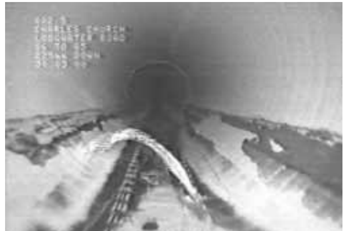
Water spray due to damage to wall of plastic pipe
